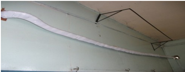
Figure 11. Location of piping
