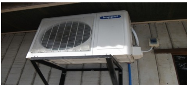
Figure 12. Location of compressor/condenser
