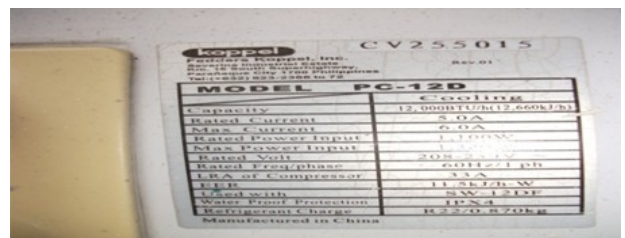
Figure 17. Actual capacity of installed ACU
