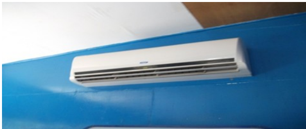
Figure 10. Location of evaporator
