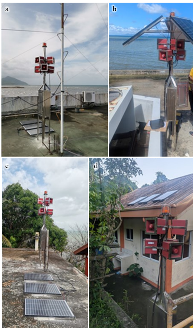
Figure 5. Installed of SIGAW units at (a) A4, (b) G4, (c) L4, and (d) C4.
